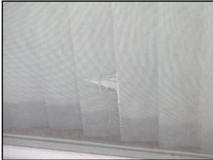
Master bedroom slider. Torn screen
