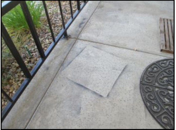
Concrete in front of bedroom 3
