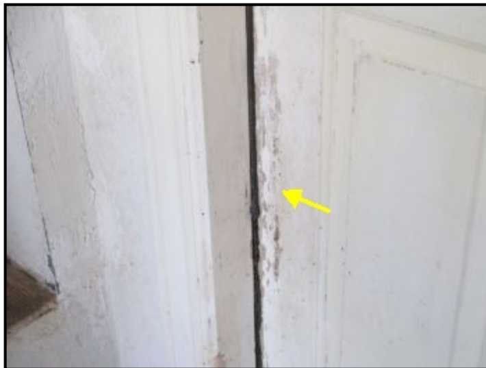
Door and weather strip damaged.
