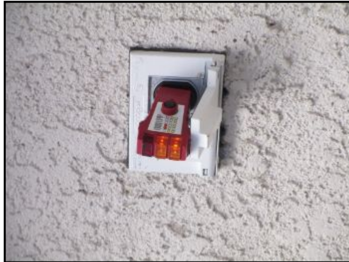
Christmas light outlet under porch
